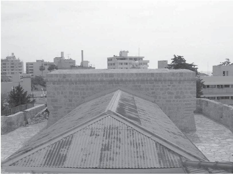
Fig. 51: Limassol Castle, roof level, chambers at the east end of the building, general view, looking eastwards [M. Olympios].
